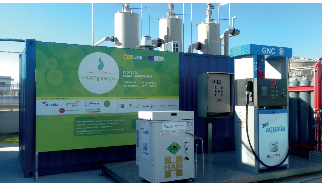
The Smart Green Gas station supplies biogas obtained from wastewater.
